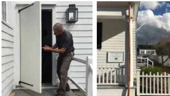
Rich Carpino, our Properties Manager, fabricated and installed a custom built board and batten door for the rear entrance of the Court House where we also cleared and replaced damaged leaders and drains for the Town.
