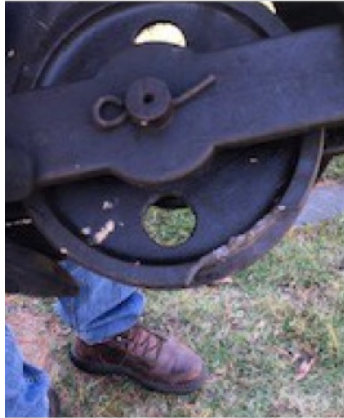
Damaged pulley discovered during disassembly
